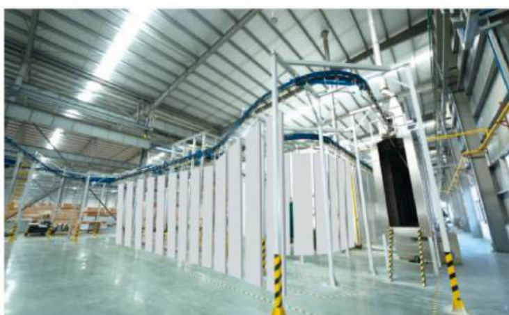
Spraying Line (German WAGNER Spraying Room)
