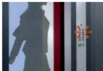
After elevator arrived, it would automatically go to the target floor, bottions for other floors would not work even if you click them.
